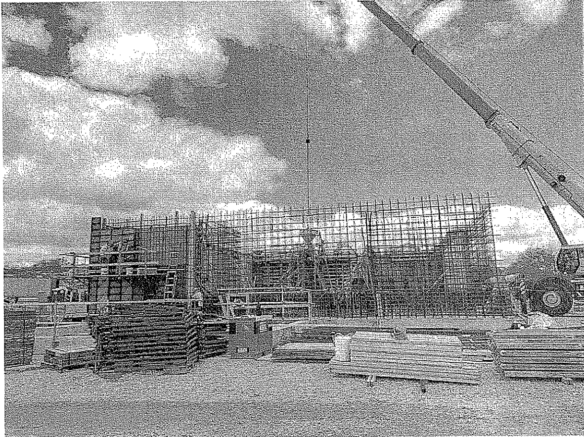
Process Building- DAF and Process Building Walls Formwork, Reinforcement and Concrete Placement
