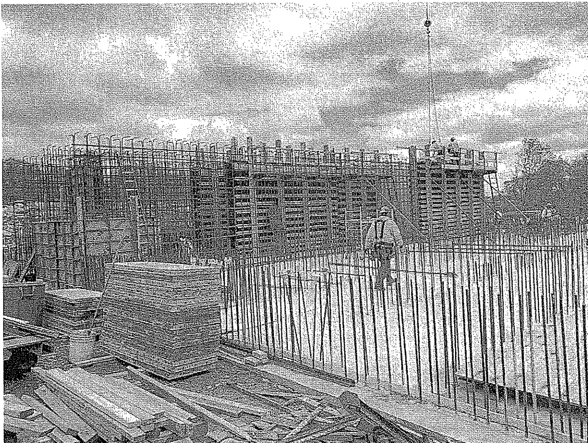
Chlorine Contact Tank - Completed South Slab Concrete and Wall Reinforcement and Formwork
