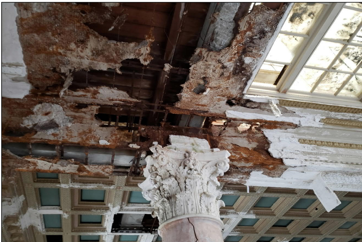
Photo 2: Typical Deterioration to Low Roof Framing Members
