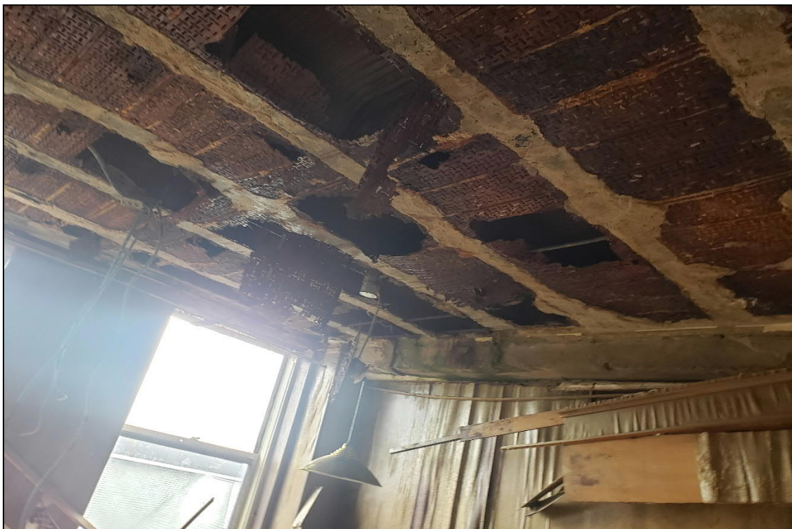
Photo 4: Typical Deterioration to Office Waffle Slab Floors
