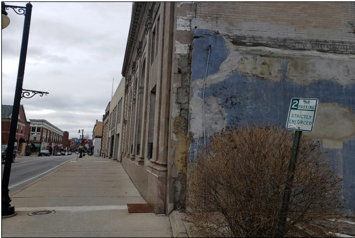
Photo 6: Moderately Deteriorated Masonry Wall at Intersection with Retaining Wall
