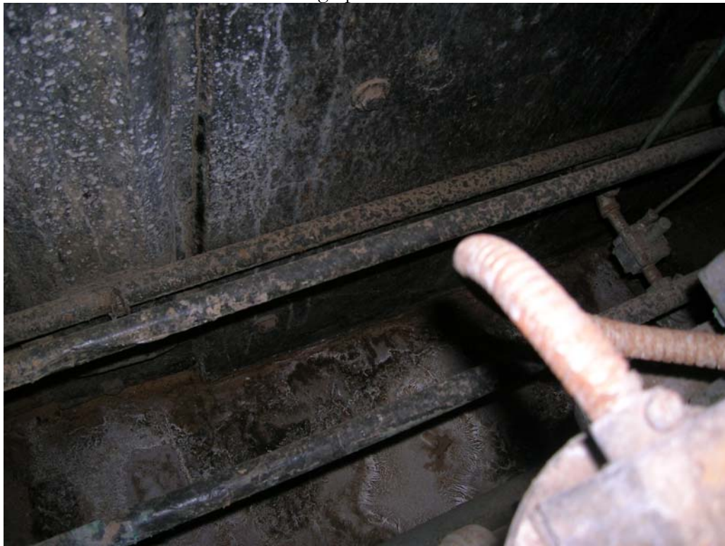
Photograph 12: Staining observed on the floor near the boilers
