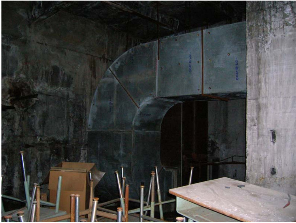
Photograph 18: Desks and heating duct in southern storage room
