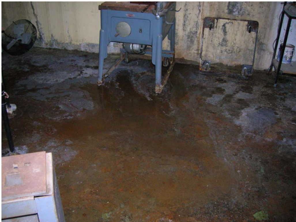
Photograph 15: Puddle of water in room to the north of the boiler room
