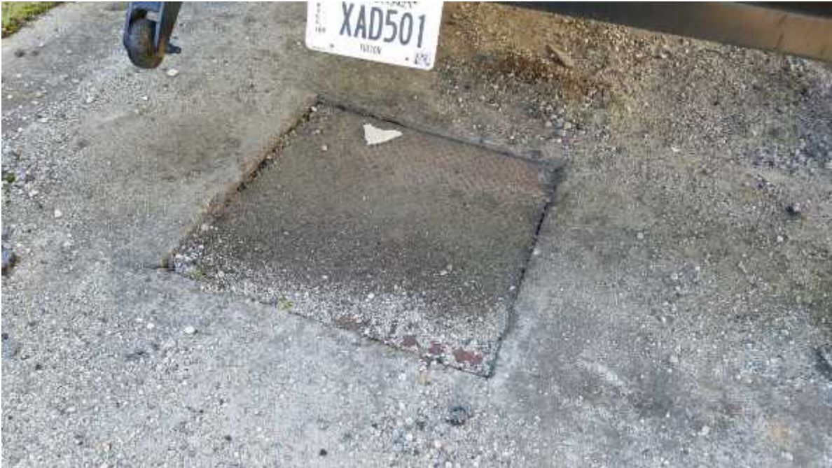
Photo 15: View of surficial indicator of a subsurface structure between the Site buildings.
