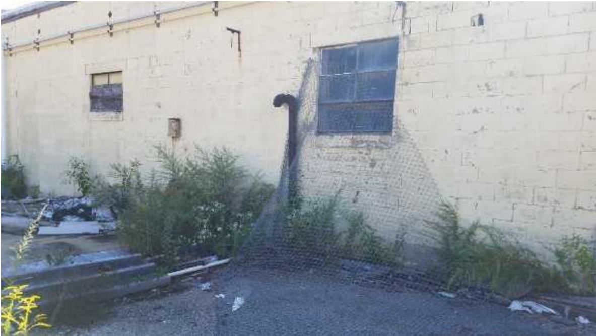
Photo 13: View of possible vent pipe for a UST along the north side of the southern Site building.
