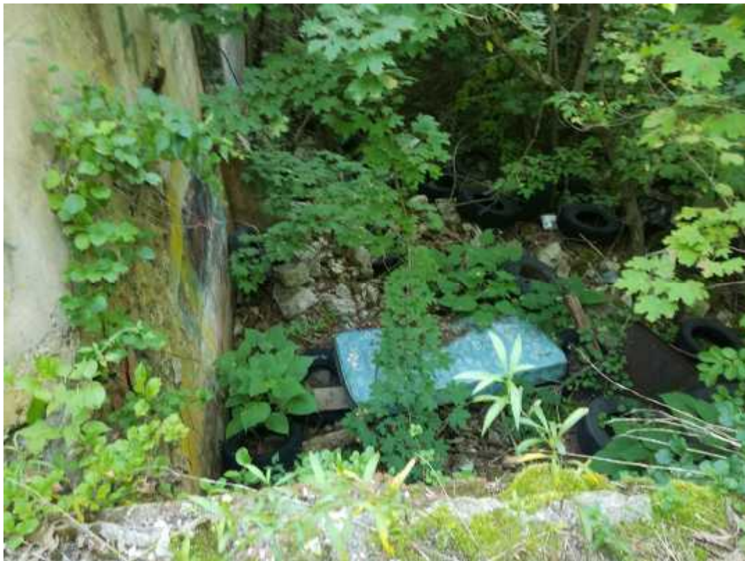
Photo 14: View looking into the foundation of the building that burned at 92 Sunnyside Avenue.
