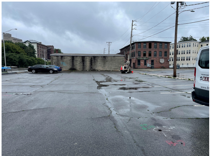
Photo shows the site looking north and the installation of monitoring well MW-3.
