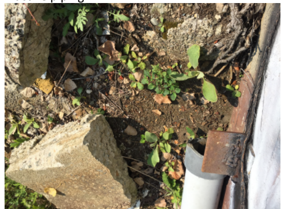
Close-up view of inactive piping.
