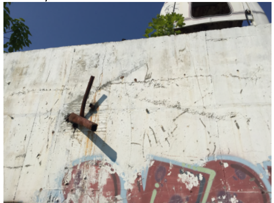
Looking west at the suspected UST concrete bunker wall and the inaccessible upper level.
