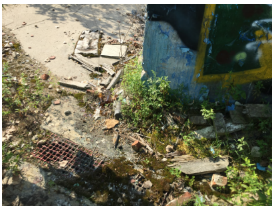
A floor grate (dry) was observed at the base of the suspected UST bunker.
