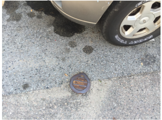
View of suspected natural gas utility cover in the roadway.
