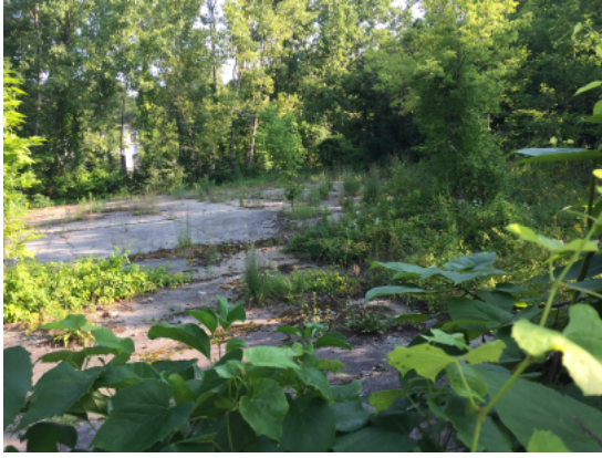
Looking northeast at cracked pavement 117 First Avenue Lot 117 containing ELUR.
