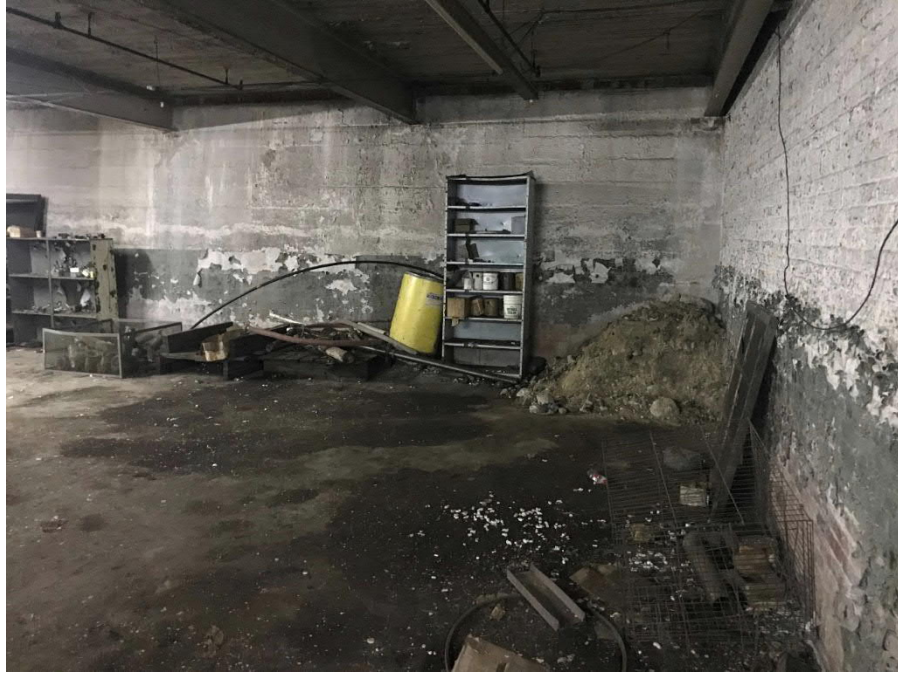
Figure 3: Floor stains, soil piles and paint cans in basement of the main building.
