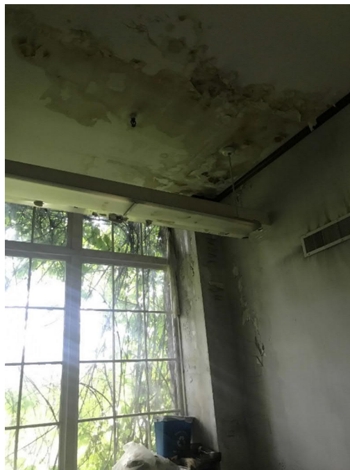
Figure 8: Mr. Moger's office ceiling on the first floor.
