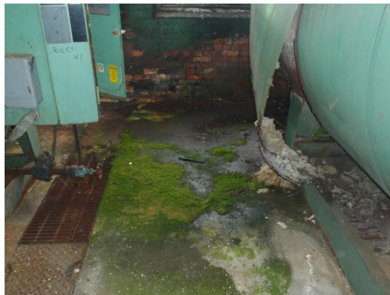
Figure 10: Moss and possible mold on first floor.
