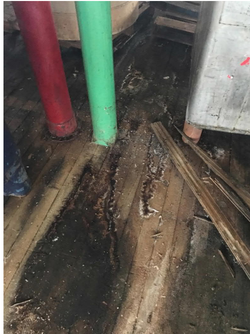
Figure 19: Dark stains on the second floor of the main building.
