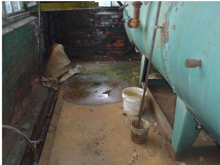
Figure 11: Rust on side of first floor boiler.
