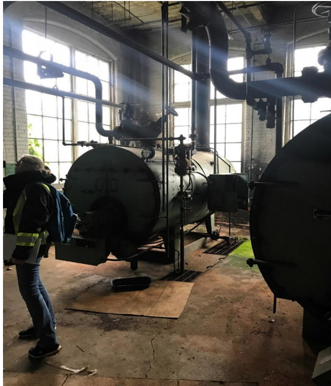
Figure 9: Two decommissioned boilers on the first floor of the main building.
