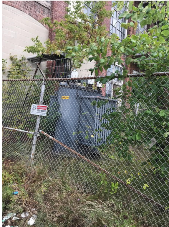
Figure 31: National Grid transformer located on the eastern side of the main building.
