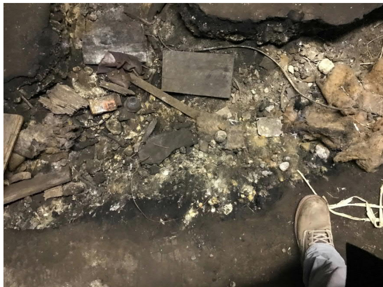
Figure 6: Miscellaneous debris in basement floor trench.
