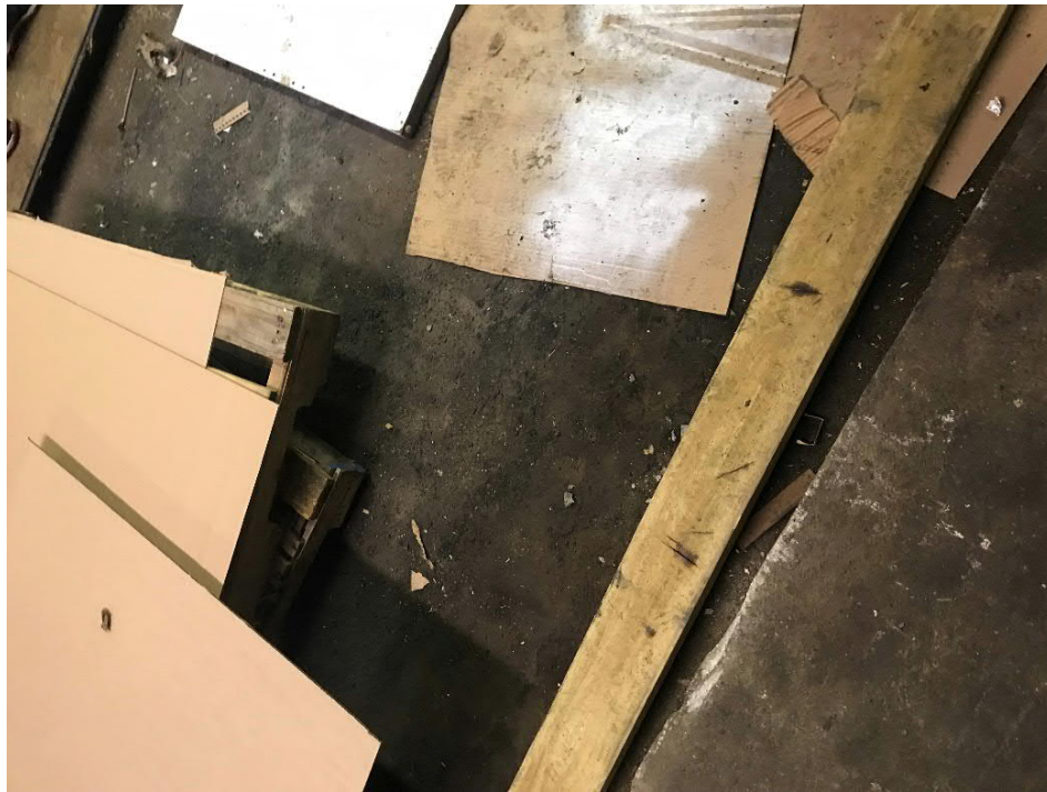
Photo 4: Exposed soil located in the first floor machine shop.
