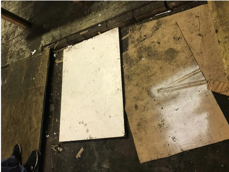
Photo 5: Exposed soil located in the first floor machine shop.
