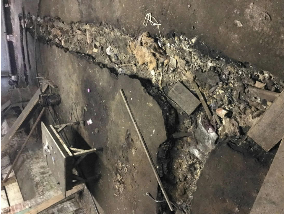
Photo 3: Exposed soil located on the western portion of the basement.
