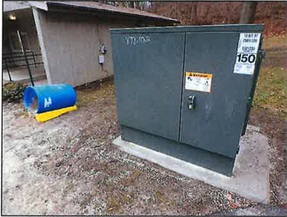
Photo 5 Photo depicting the configuration of the new transformer and concrete pad, as viewed from the east.
