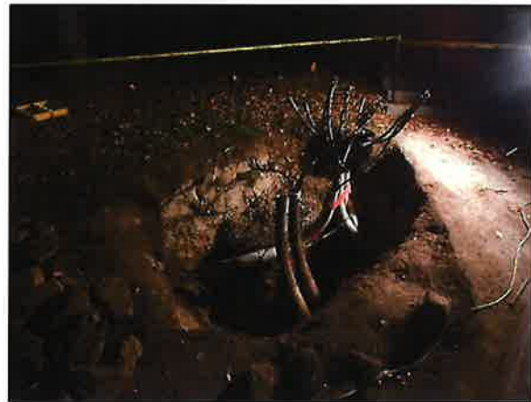
Photo 4 Site conditions subsequent to the completion of response actions, as viewed from the southeast.
