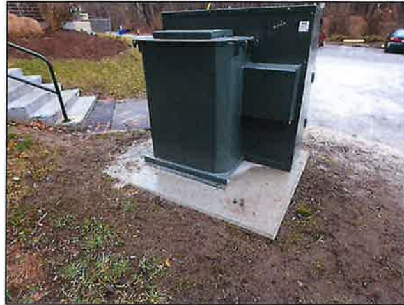
Photo 6 Photo depicting the configuration of the new transformer and concrete pad, as viewed from the west.
